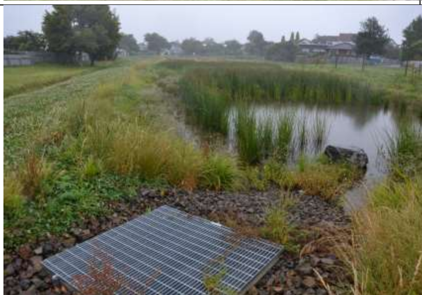
Submerged outlet pipe with connection to hydraulic controls within grated manhole
