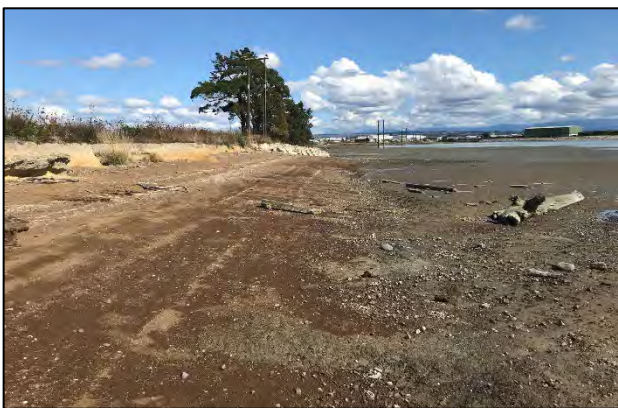
Erosion near Saxton Creek
