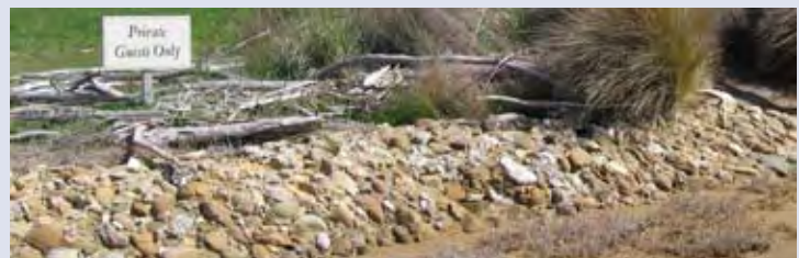
Small seawall constructed to protect residential land from erosion.
