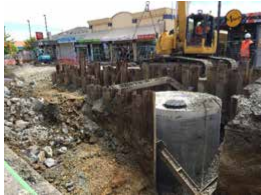
Figure 7: Flood mitigation is expensive - photo Queen Street project
