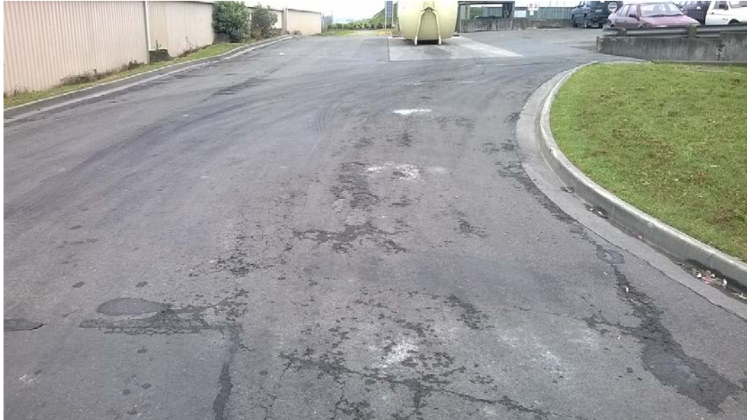
Figure I-4: Example of Aged Chip Seal Suffering from Scabbing and Cracking
