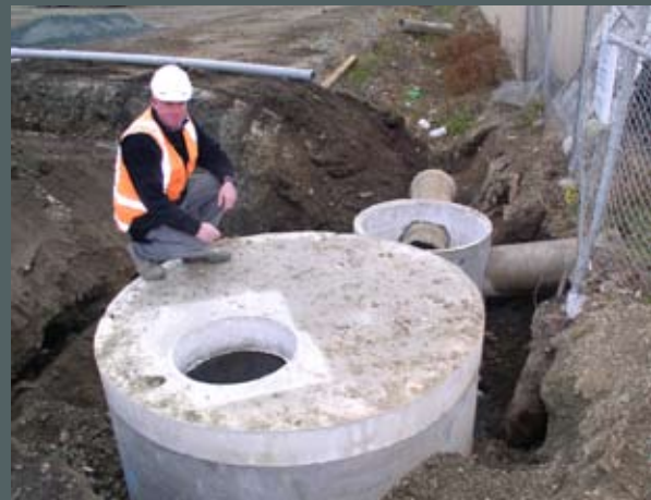
Beach Road humes interceptor.
