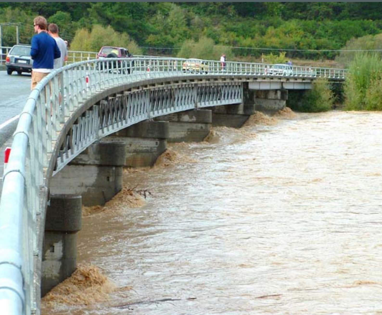
Kohatu Bridge during flood.
