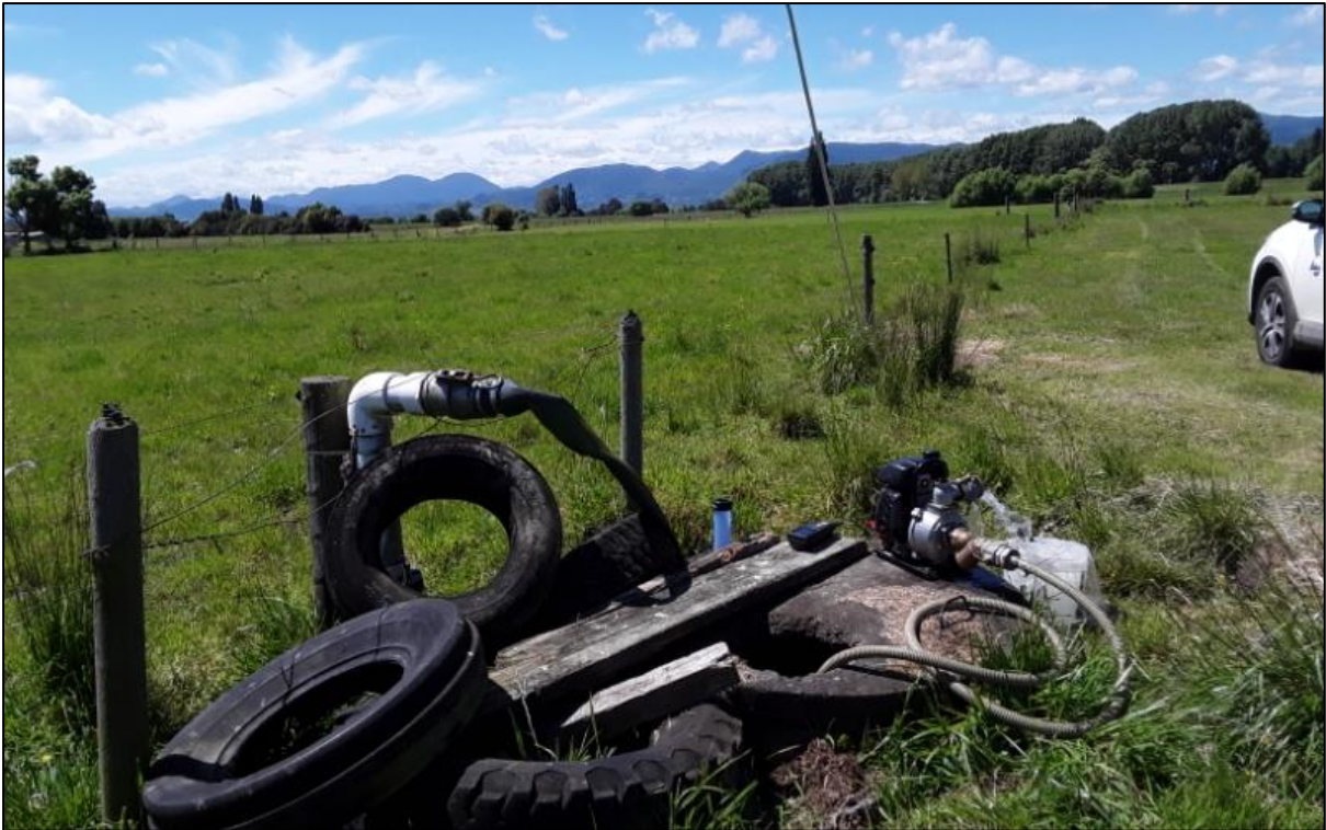
Figure 6: Well with no adequate well head protection. Contamination can easily enter into the groundwater by falling directly into the well.
