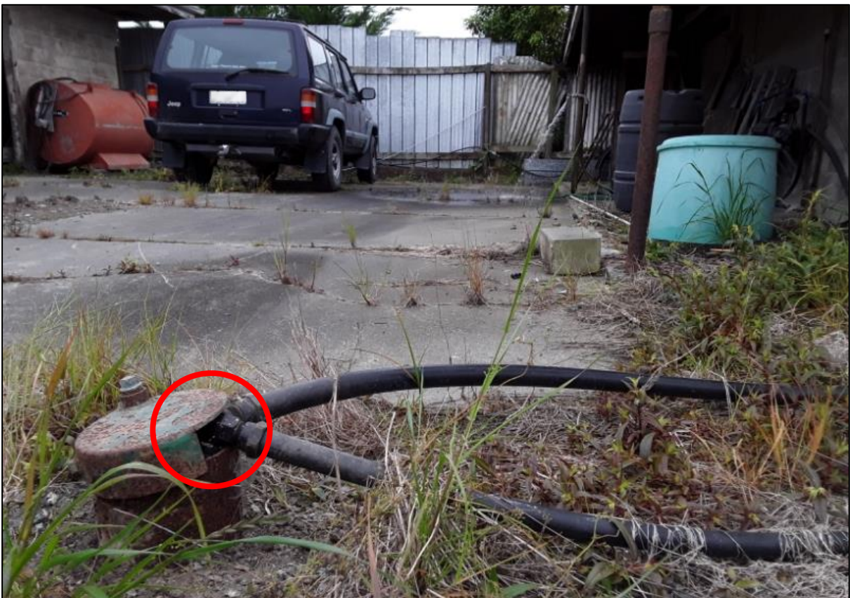
Figure 7: Bore located in low lying area without adequate bore head protection. Contamination can easily enter into the groundwater from the bore.
