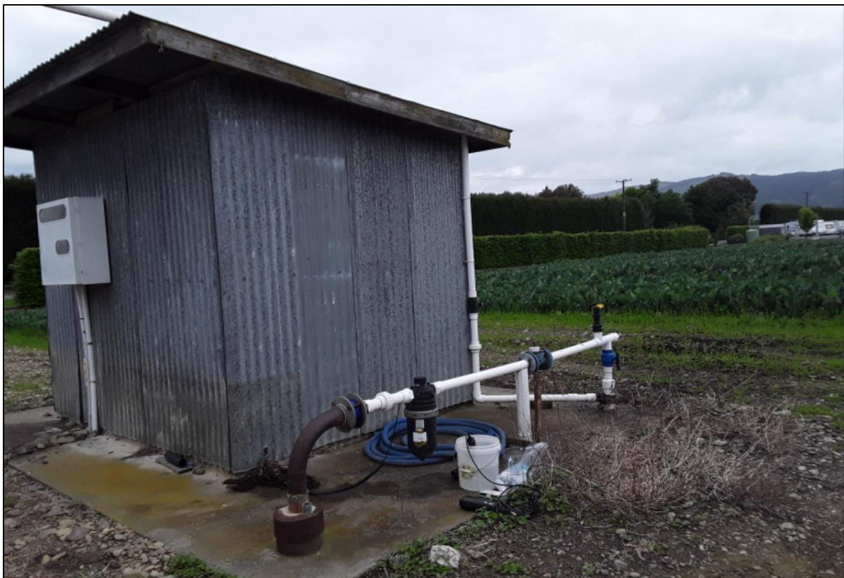
Figure 8: Bore with a sealed bore head located above the ground to prevent stormwater runoff entering the bore. Backflow prevention device installed to prevent contaminated water flowing back into the aquifer. Concrete pad to deflect stormwater and prevent direct soakage into the bore.
