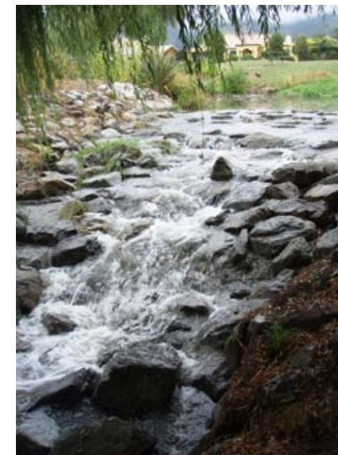
A rock ramp on Reservoir Creek at the Templemore Pond outlet is more fish-friendly than the previous vertical concrete ford
