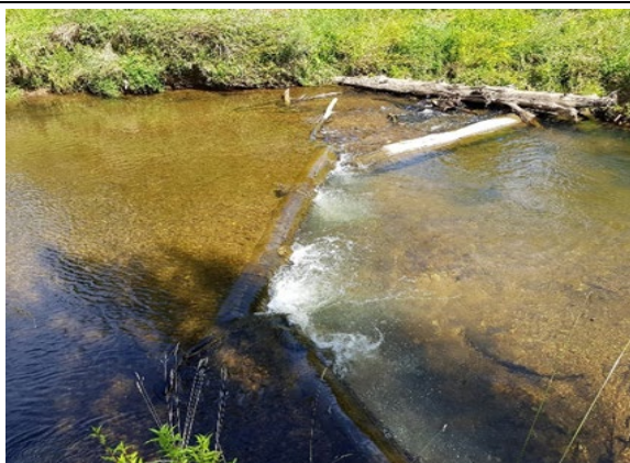
An example of a cross-vane weir constructed from wood and anchored using a duckbill anchor (image from WRC unpublished).
