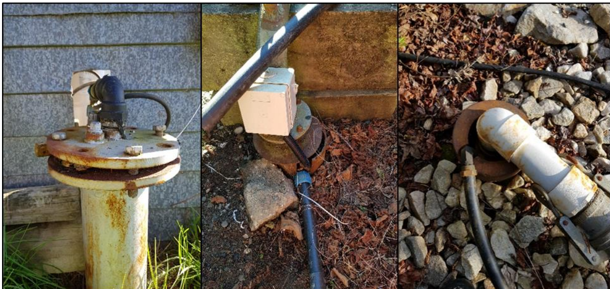
Figure 12: Examples of modified or poorly sealed boreheads from the 2019 Motueka / Riwaka Plains survey.
