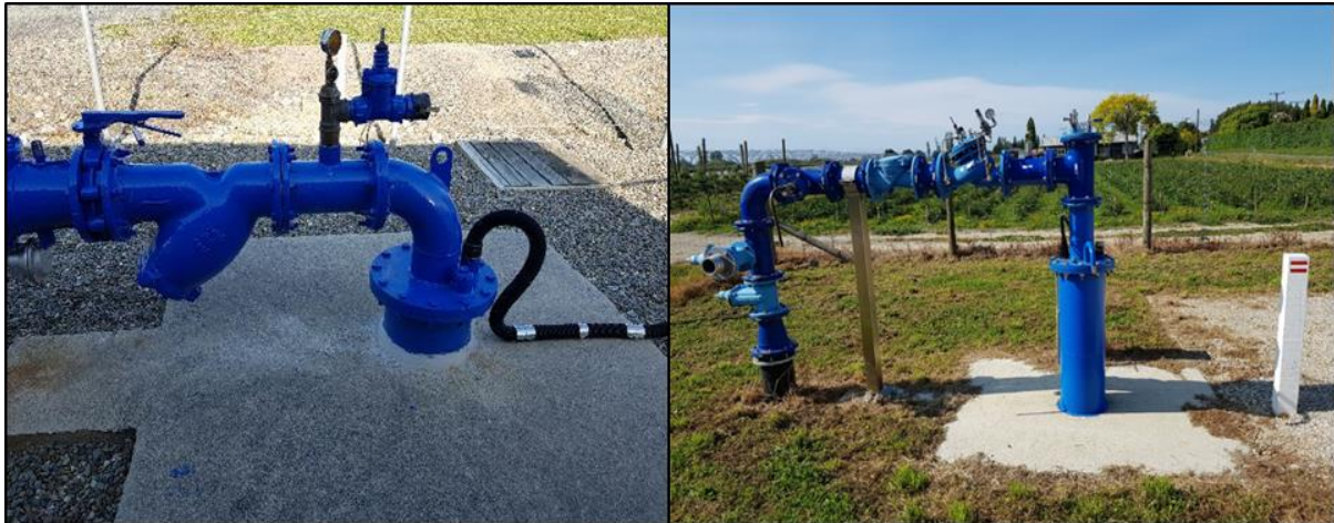
Figure 11: Examples of Council reticulated water supply bores from the 2019 Motueka / Riwaka Plains survey.
