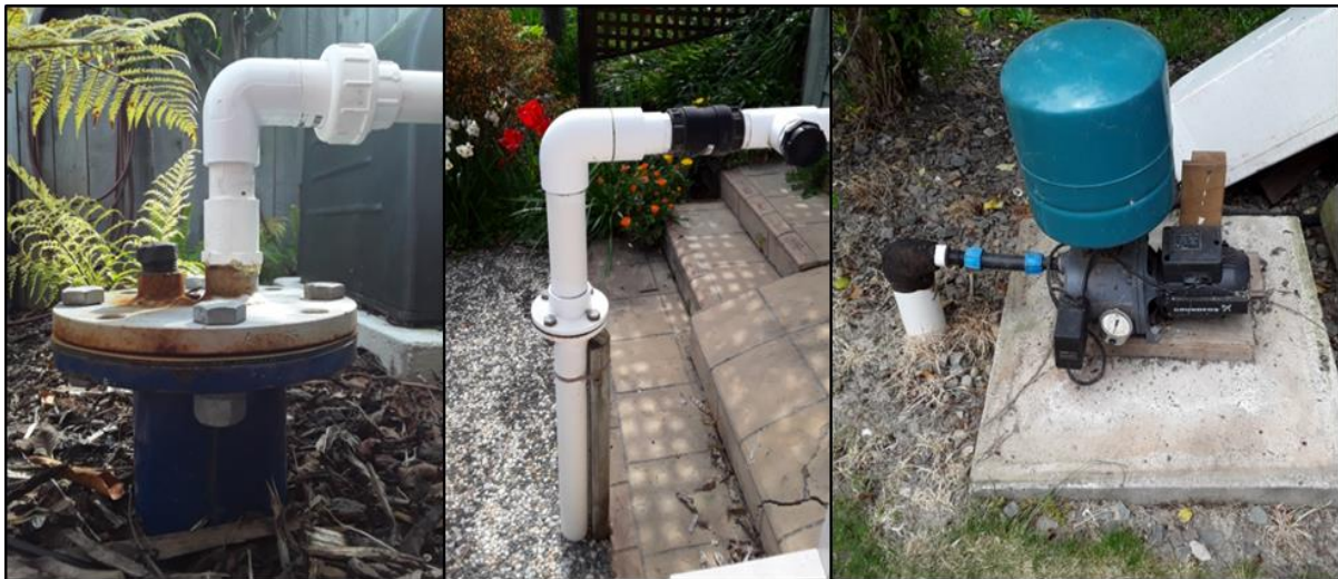
Figure 15: Examples of good private boreheads / practices from the 2019 Motueka / Riwaka Plains survey.
