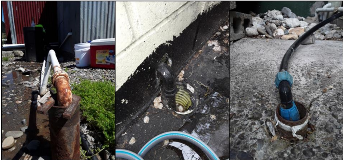
Figure 13: Examples of poor private boreheads / practices from the 2019 Motueka / Riwaka Plains survey.
