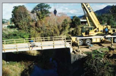
3. Latest new bridge – A third dairy raceway bridge under construction at Matariki on the Sherry River (May 2003).
