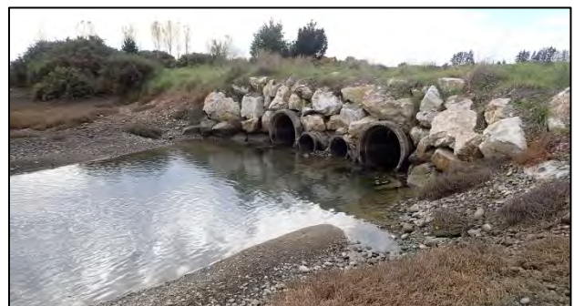
Moon Creek culverts under Thorp Street on the western estuary margin
