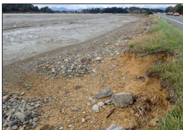
Eroding and unvegetated road margin
