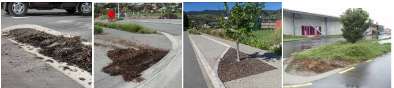
Narrow bioretention and small cell on corners with no protective edges are highly vulnerable to traffic damage
