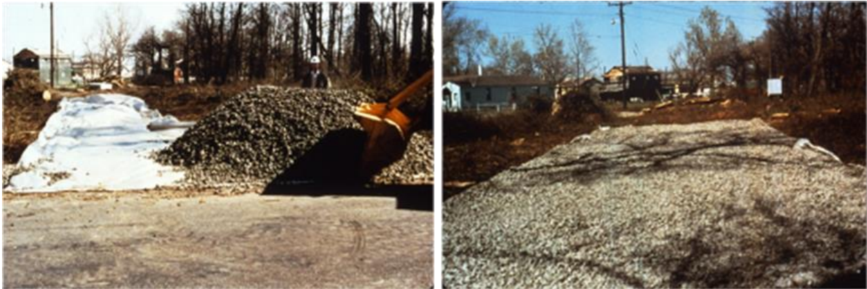
Figure 8-19 Stabilised construction entrance showing progression of construction with filter fabric underlay prior to stone placement
