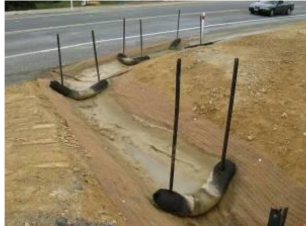
Figure 8-2 Fabric filled check dams in conjunction with erosion control matting. Note flow evidence over the centre portion of the dams
