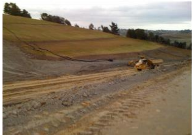
Figure 8-5 Contour drains established on embankments as a water control measure in conjunction with progressive stabilisation.
