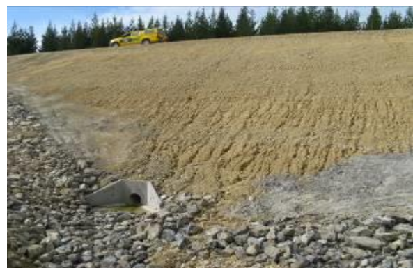
Figure 3-7 Rill Erosion on a Highway Embankment
