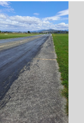
Surface cracking (new):
