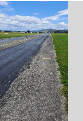
Surface cracking (new):
