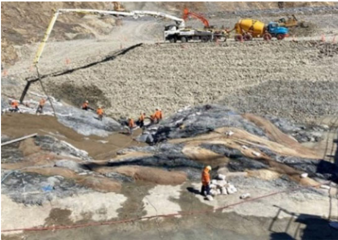
Figure 7: Defect treatment of third Embankment foundation
