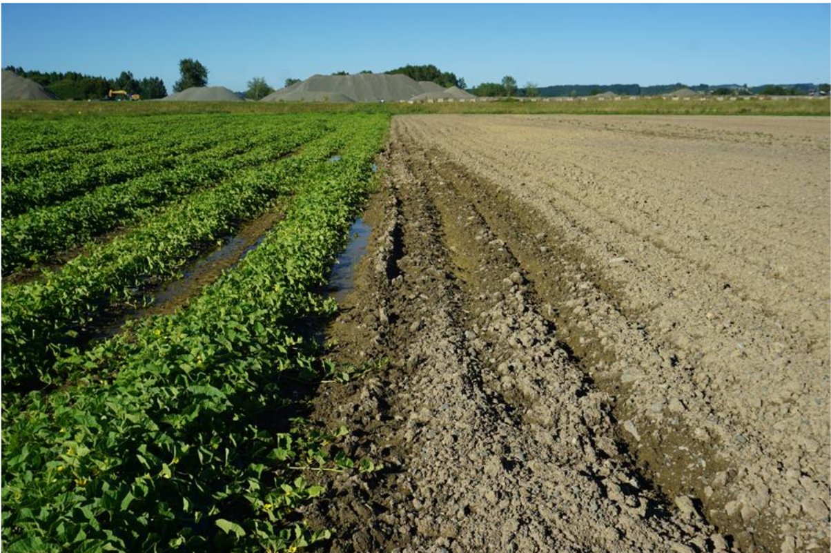
Figure 4 – Example of surface depressions in reinstated soil (year two to the left, and year four to the right).
