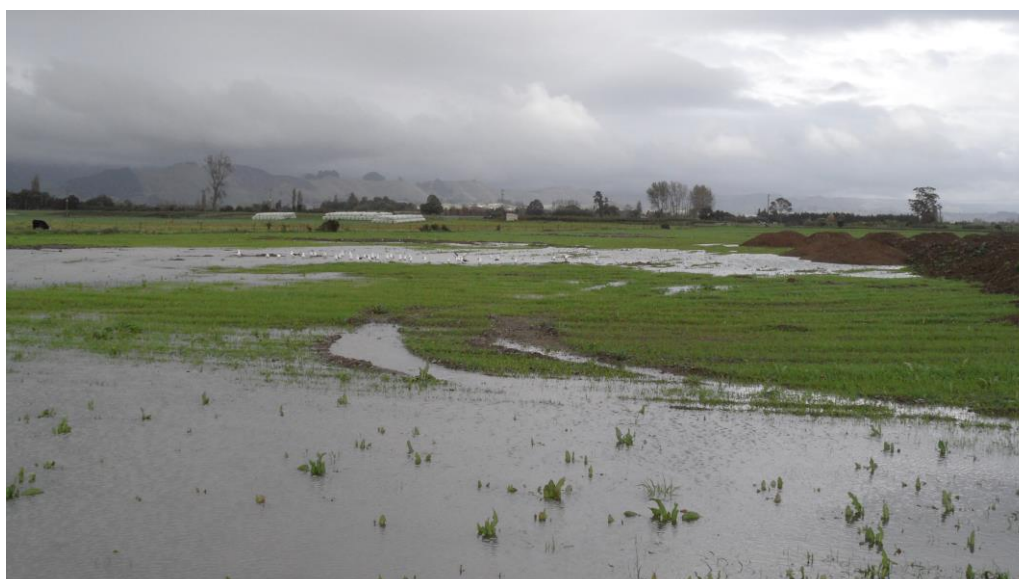
Figure 13. Water ponding on restored land.
