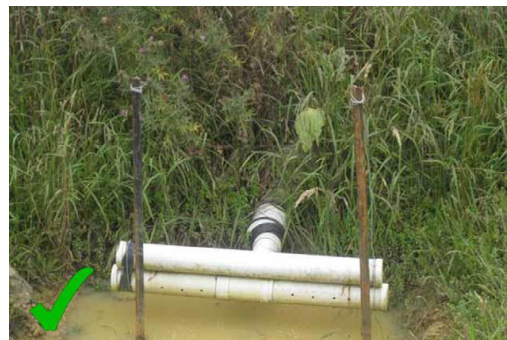
Figure 9-18 Floating Decant in DEB
