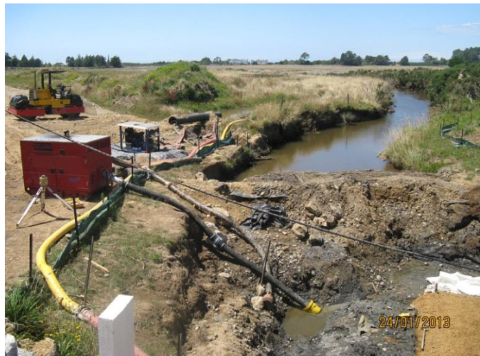
Figure 11-1 Bridge construction with a temporary stream diversion using pipe (yellow) and pump (not shown). The pump shown is dewatering the works area to an offline sediment retention pond)
