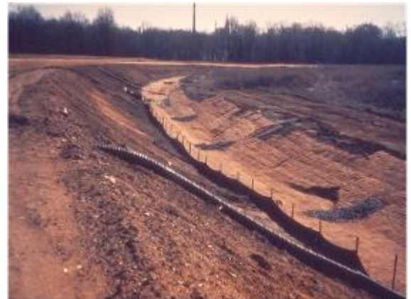
Figure 8-12 Pipe drop structure (note check dams, silt fence and channel protection also)
