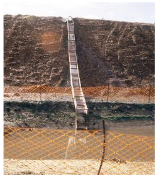
Figure 8-13 Flume to a sediment retention pond
