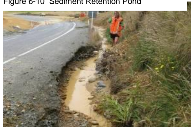
Figure 6-11 Storm damage needing new management and repair
