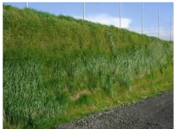
Figure 8-236 Hydroseed being applied to a vertical face and the eventual stabilisation (photos courtesy of Erosion Control Ltd).
