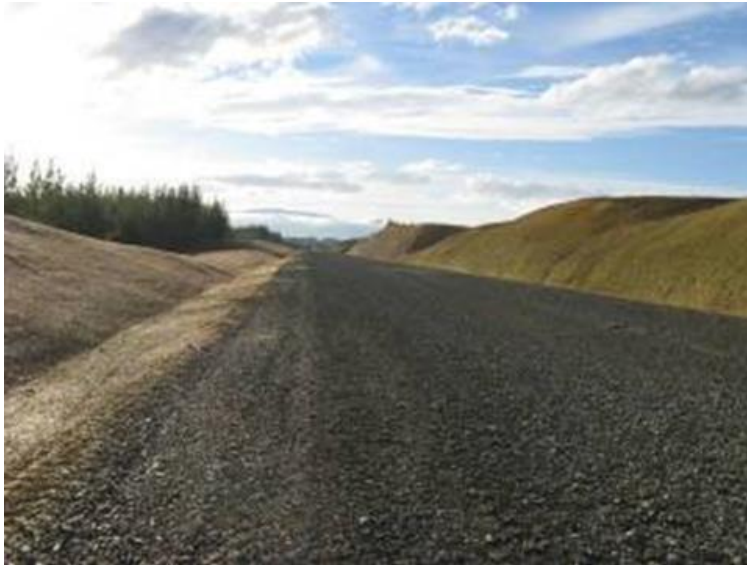
Figure 6-5 Good Example of Straw Mulch, Temporary Seeding and Aggregate Stone to Limit Exposed Area
