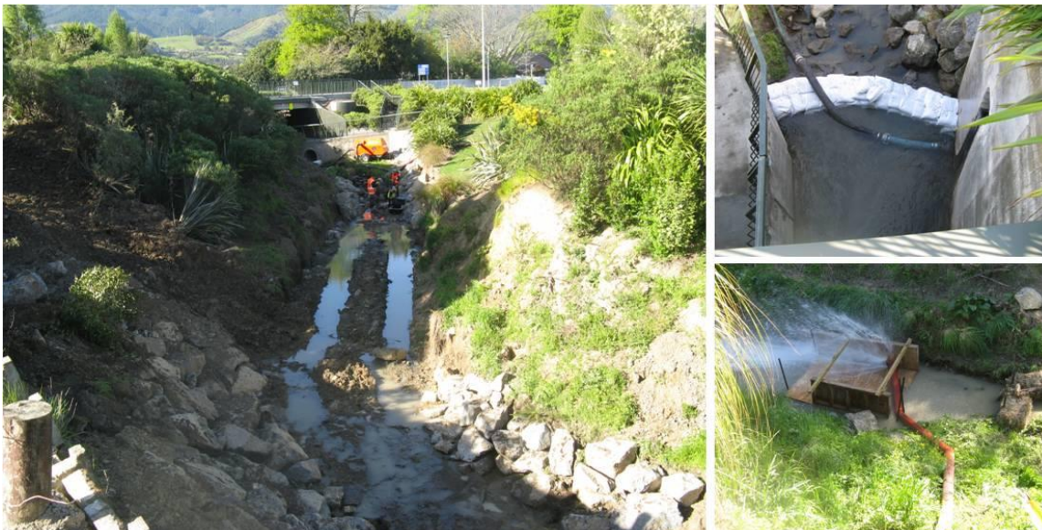
Figure 11-12 Reservoir Creek diversion with intake pipe (upper right) and outlet with energy dissipation (lower right)
