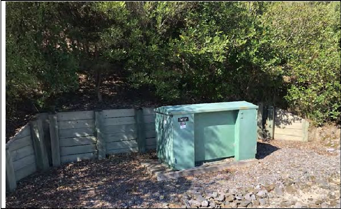
Photo 9: 400v Underground Mains Power Transformer
