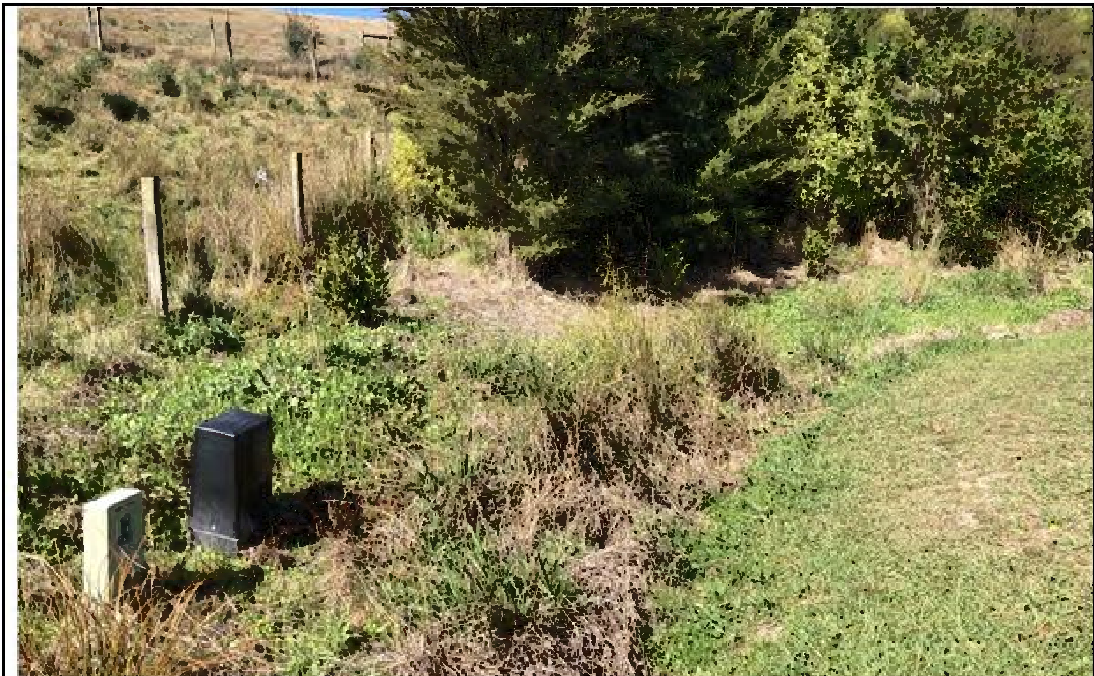
Photo 10: Fibre Optics Telecommunications Infrastructure
